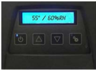
Local Interface Controller
